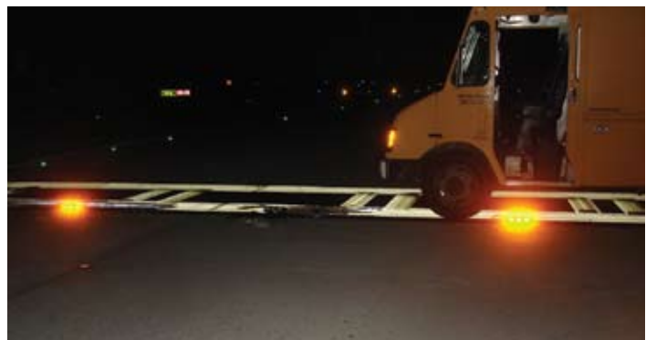
Figure E. Installed L-852G LED Fixtures.
